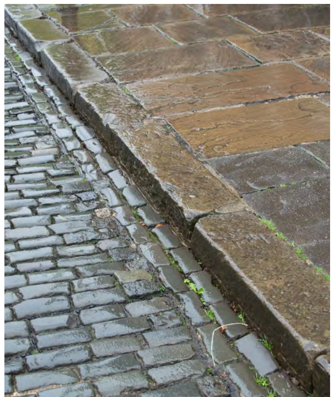
Walk around or inspect your premises to identify slip and trip hazards.
