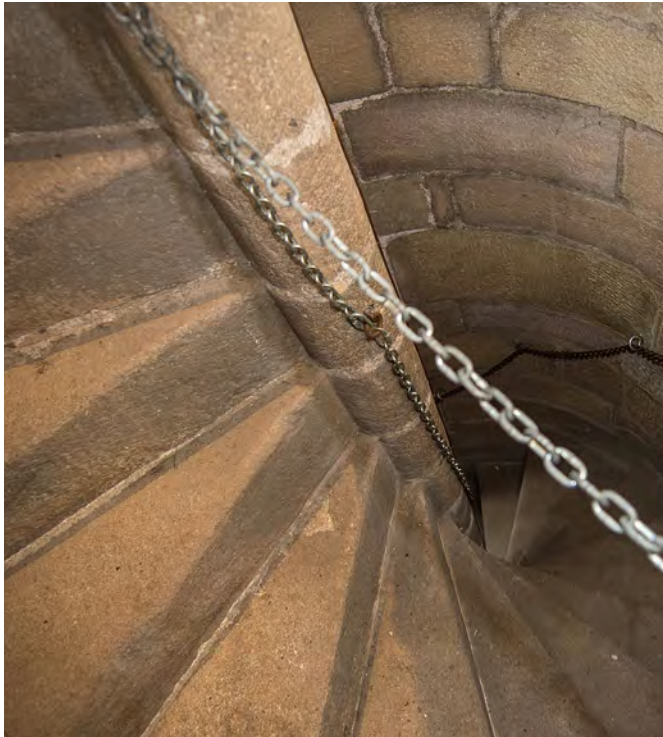
Risk assessments should consider slips and trips on stairs including areas not accessed frequently.
