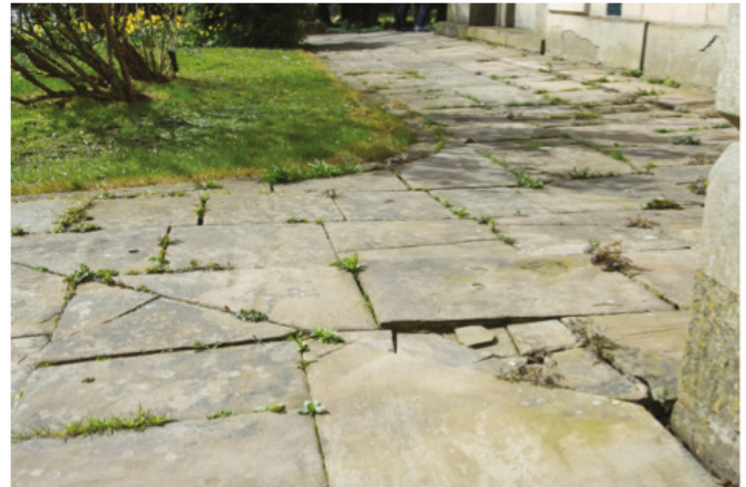
Broken paving should be noted during routine maintenance checks and suitable precautions taken until any damage can be repaired.
