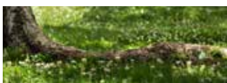
Protruding tree roots and undergrowth particularly on footpaths or other access routes
