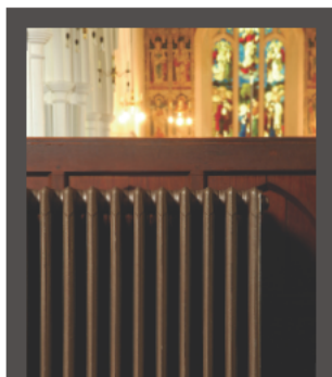
All heating apparatus should comply with the relevant British Standards and Building Regulations.
